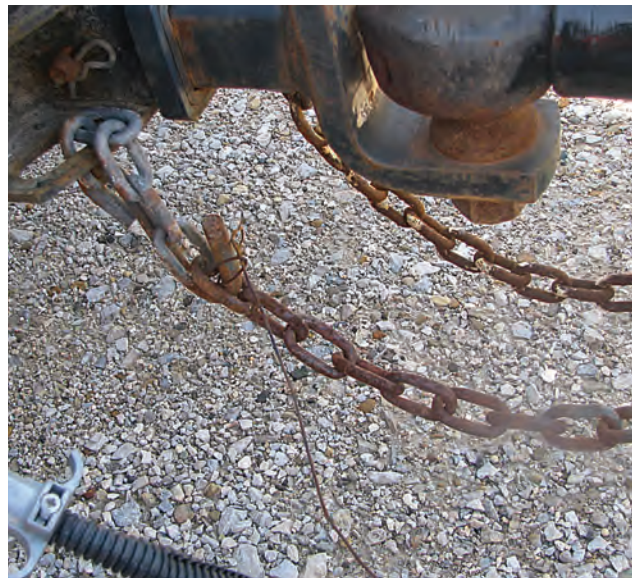
The wire is so rusted that it would pull apart before it could activate the emergency brake.
